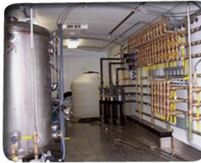
Photo of one of the dozens of groundwater recirculation trailers designed, constructed and installed by IESI.
