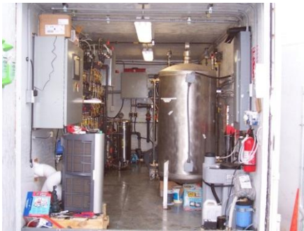
Photo of one of the dozens of groundwater recirculation trailers designed, constructed and installed by IESI.
