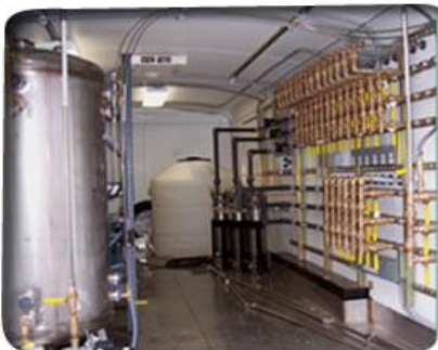
IESI has designed and constructed dozens of Groundwater recirculation trailers.
