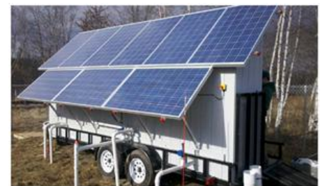
Photo of a solar powered remediation trailer for 1,4 dioxane.
