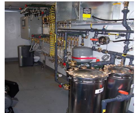
Above are photos of the interior of Remediation system trailers.
