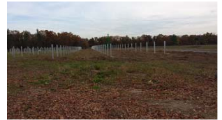
Above is a construction process photo of IESI's latest 4.9 MW project in Southwick, MA.
