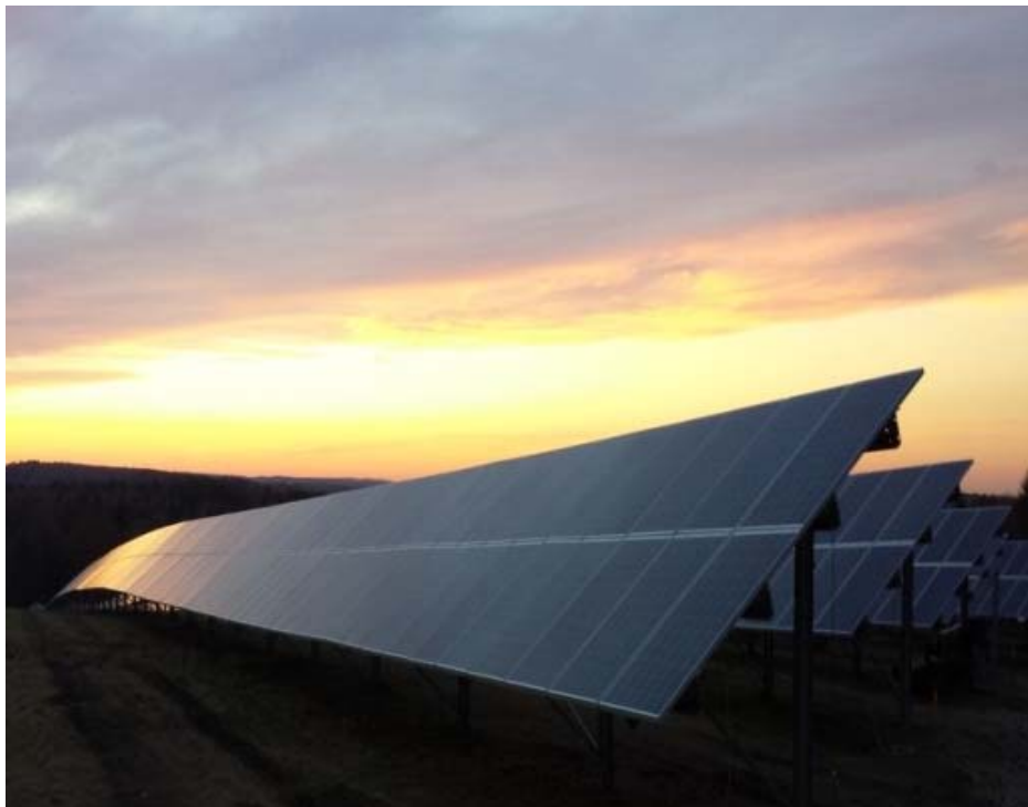
SOLAR POWER IS A BEAUTIFUL THING!!! (PHOTO FROM IESI PROJECT SITE)
